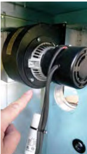
1.19 Check operation of new exhaust fan.
